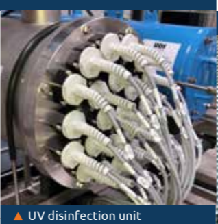
▲ UV disinfection unit
