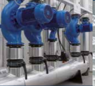
▲ cold water distribution
