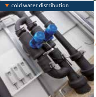
▲ irrigation valve set
